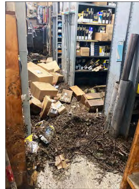
Flood debris fills a shop at Bear Mountain State Park. (Photo provided by Daniel Corigliano.)
