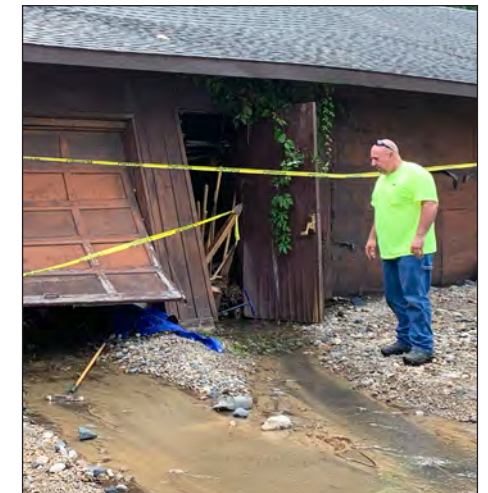
A stream now flows through the condemned building that once housed Cristian Gonzalez’s Carpentry shop.
